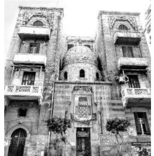
Figure 9. Deterioration of heritage buildings (Mausoleum of Sidi Yacoub)
