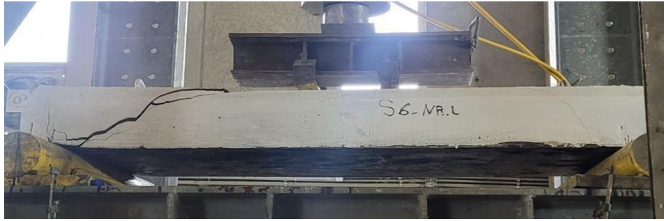
Figure (4 to 6) Crack patterns of Slabs (S1to S6)
