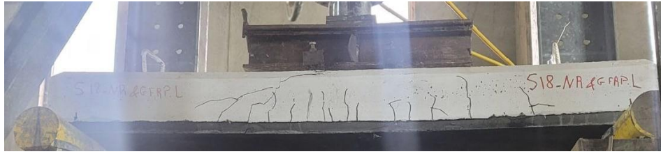
Figures (13 to 18) Crack patterns of Slabs (S13to S18)
